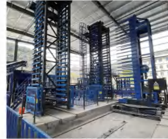
HIGH POSITION CURING ROOM SYSTEM
